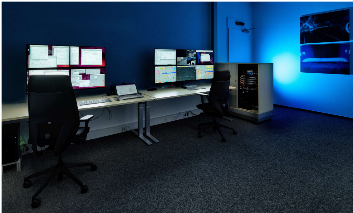
Figure 11: Scientific workstation and control display panels in the control room
